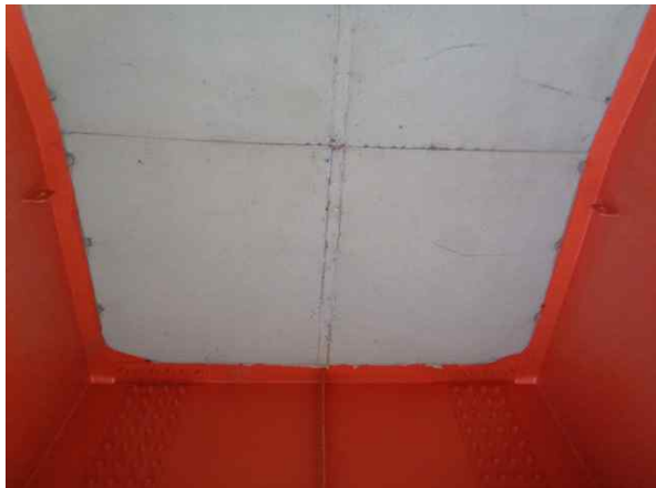
S6 균열 (0.2mm/2.0m)
