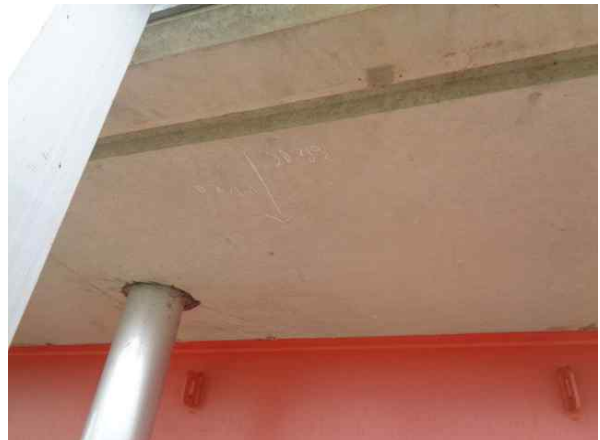
S1 캔틸레버부 균열 (0.2mm/1.0m)
