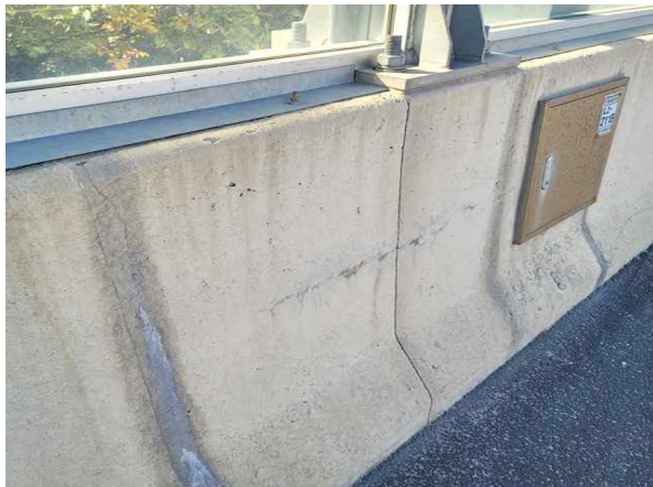
S1 균열 (0.2mm/1.0m)
