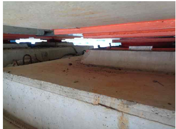
P5-Sh12 받침물탈 파손 (0.1m×0.1m)
