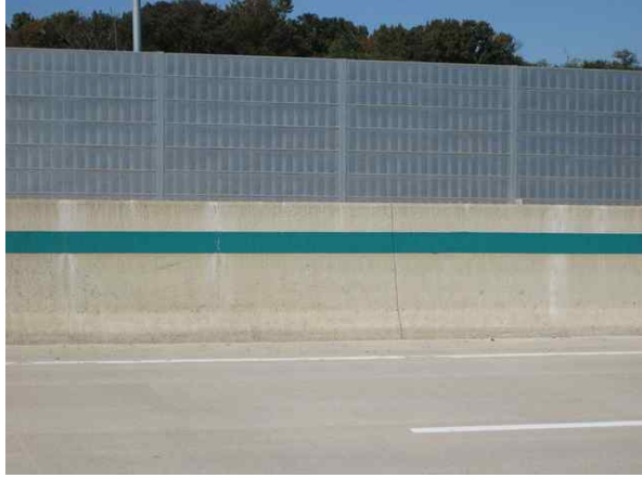
S3 방호벽 균열(0.2mm/1.5m)
