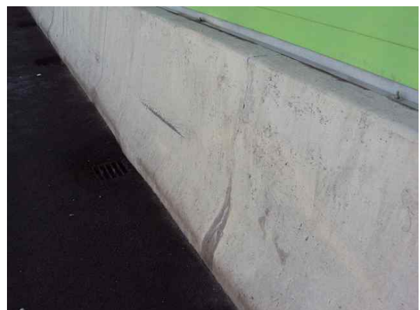
S5 방호벽 균열 (0.2mm/1.2m)
