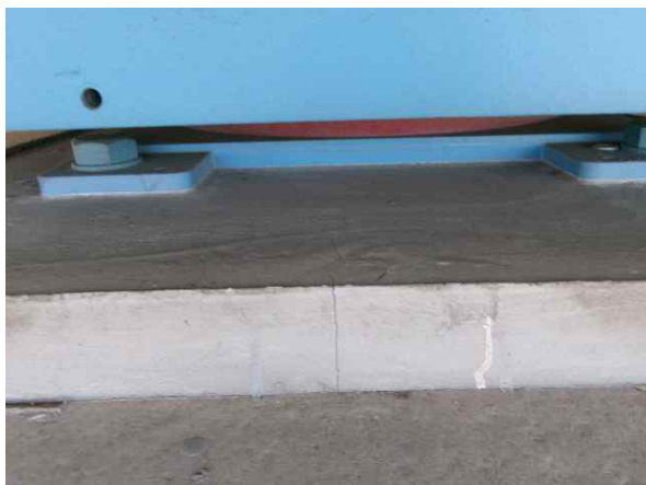
P2-Sh3 받침몰탈 균열 (0.2mm/0.2m)
