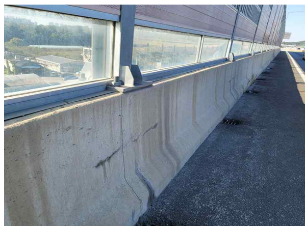
S6 균열 (0.2mm/1.5m×12EA)
