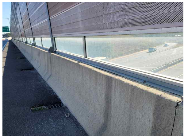
S2 균열 (0.2mm/1.5m×14EA)
