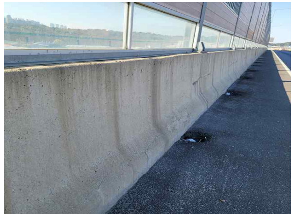
S5 균열 (0.2mm/1.5m×24EA)
