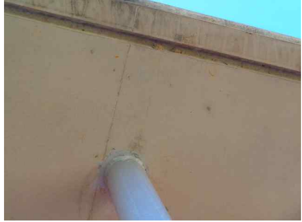
S1 캔틸레버부 균열 (0.2mm/1.0m×2EA)
