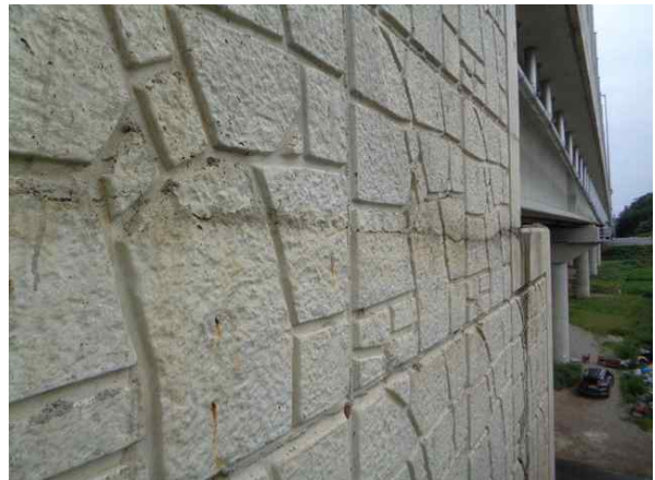
A2 균열 (0.2mm/3.0m)
