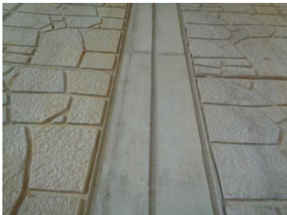
A2 균열 (0.2mm/5.5m)
