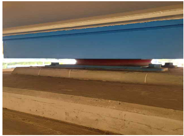
P1-Sh2 받침물탈 균열 (0.2mm/0.4m×3EA)
