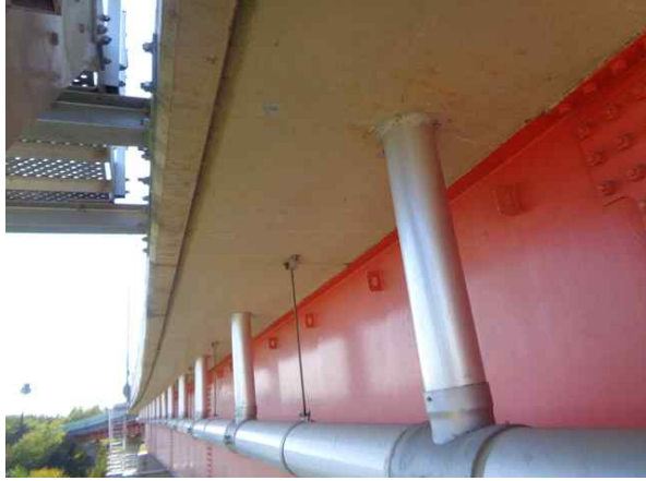
S1 캔틸레버부 균열 (0.2mm/1.0m×2EA)
